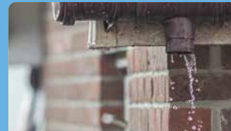
Broken or blocked guttering
